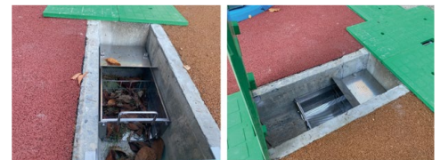
MP Filter when installed
