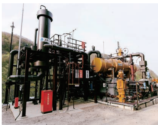
Binary geothermal power plant
