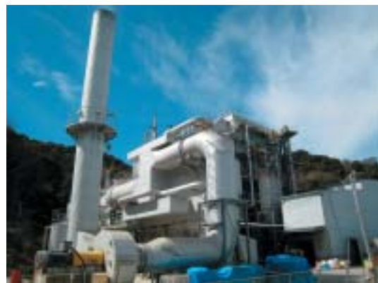
Source: NANGOKUKOSAN Co., Ltd.
