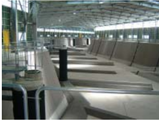
Example of final disposal site with roof (Takasaki General Waste Final Disposal Site in Miyakonojo-shi) Source: Research Committee for Closed System Disposal Facilities
