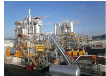
Temporary incinerator in Kesenuma city, Miyagi (2012.12.23)
