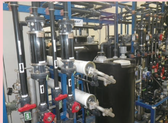
Photo 1 Pilot plant introduced in Itoman City Sewage Treatment Center (Photo credit: Yoshikatsu Nakano)
