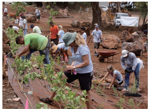
Photo 10. In Wahikuli, West Maui in Hawaii, members of the regional council and volunteers are planting through united efforts an endemic species on the slope as a measure for preventing sediment runoff. (Provided by West Maui R2R)
