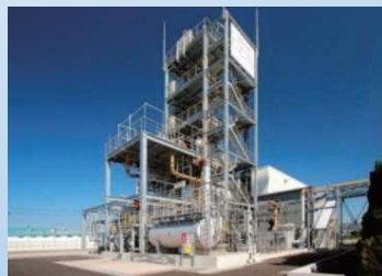
Facility to capture CO2 emissions from power plant (from MOEJ website)
