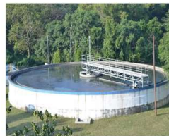
Kalyani 21 MLD NJK (STP)
