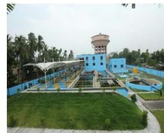
Bhatpara 41 MLD NJK (STP)
