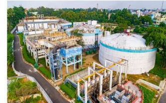
Pahari, Patna 60MLD NJK (STP)
