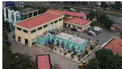
Nhieu Loc - Thi Nghe Wastewater Treatment in Binh Thuan District of HCMC
