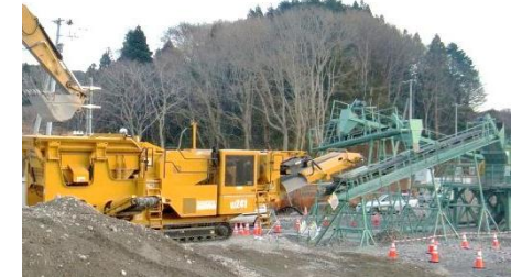
Treatment facility for concrete debris in Yamada town, Iwate (2012.12.11)
