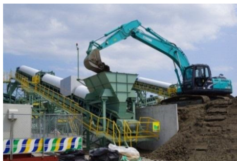
Treatment facility of tsunami deposit in Rikuzentakata city, Iwate prefecture (Test operation from May 7, 2013)
