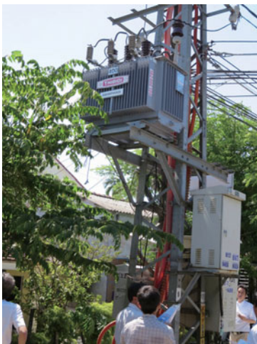
Amorphous Transformer Installed in Ben Tre Province
