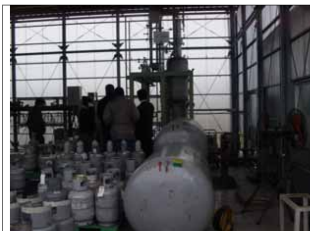
Reclamation facility (for gas refrigerant)
