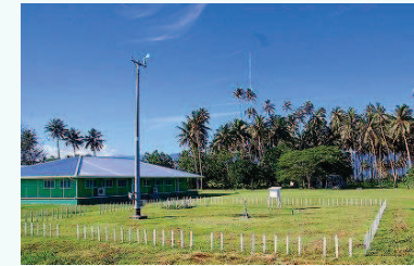
Equipment installed at Samoa meteorology headquarters
