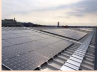
Solar power generation facilities
