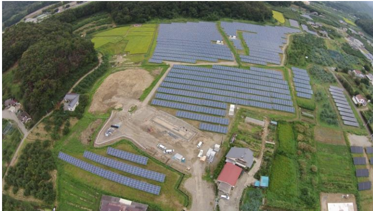
Large-scale solar power generation facility in Fukushima City (Photograph provided by Apollo Gas Co., Ltd.)
