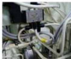
point: hose joint 59. 4L/min
