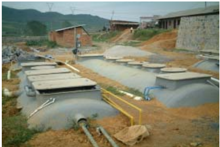
Photo 7-1-3 Medium-sized private sewerage system
