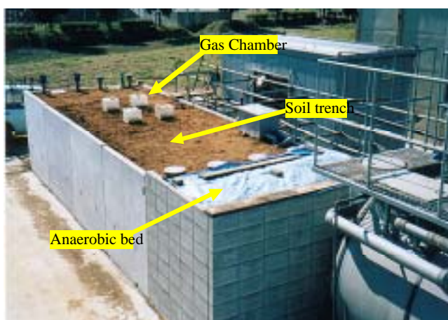
Photo 6-1-2 Soil treatment system experiment equipment installed at Kokinu Experiment Site
