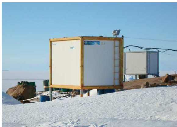
Figure 4.1 Diesel generators at Mount Vechernyaya field base
