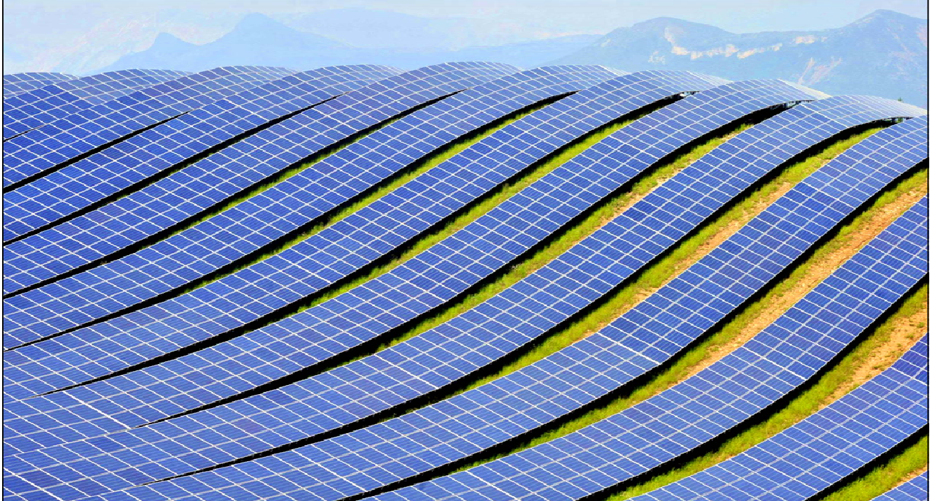
30.94 MW Solar Park, Le Mees, Alpes-de-Haute-Provence, France http://time-az.com/main/detail/31458
