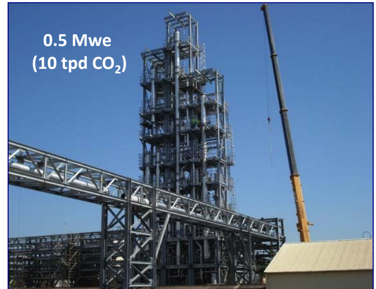
Pilot Solvent Test Unit (PSTU)
