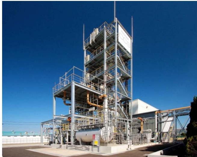
Post Combustion CO 2 Capture Pilot Plant (Toshiba)
