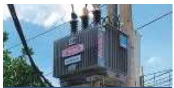
Amorphous transformers in power distribution, Yuko-Keiso, Vietnam
