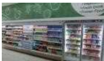
Energy saving at convenience stores, Panasonic, Indonesia
