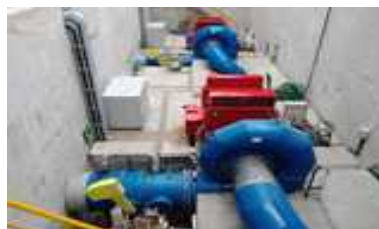
Hydro Power Plant, Toyo Energy Farm Co., Ltd., Indonesia
