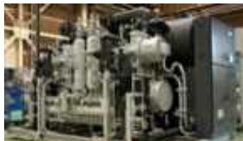
High-efficiency refrigerator, Mayekawa MFG, Indonesia
