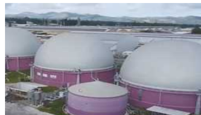
Biogas Power Generation, ITOCHU Corporation, Philippines
