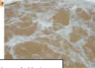
Aeration tank, No.1
